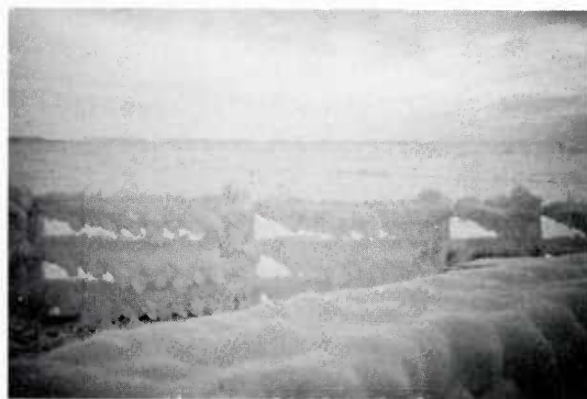
Figure 2-1 Guard rail ice accumulation.
